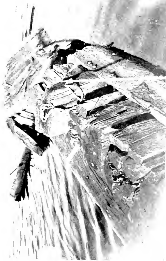
2711. One of the heavy beams of the two-decked, iron-hulled, barkentine schooner, Henry T. Hood , which was damaged April 17, 1914, and is now on the pier at Sackett's Harbor, opposite the Shiphouse Point.
